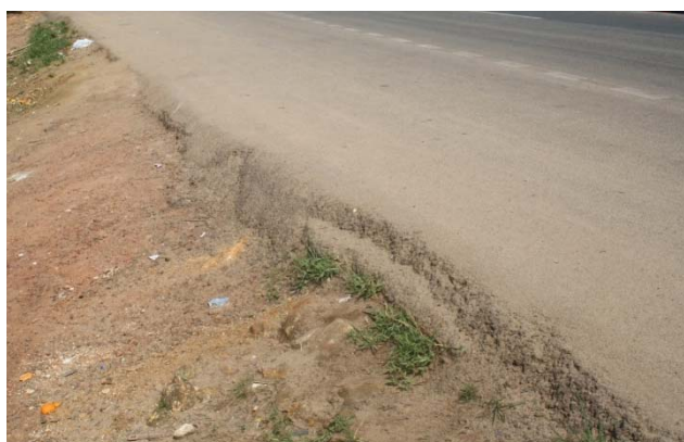
Plate 1 Edge Drop at Kareelakulangara Junction
